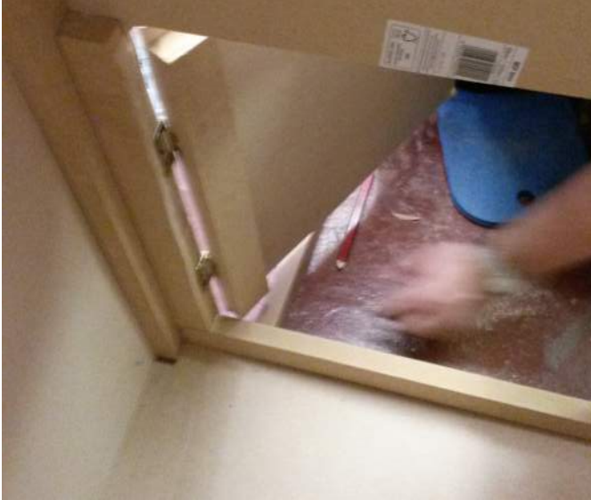
Step 10: The square cut for the door opening was then used as the door using timber to reinforce and hinges.
